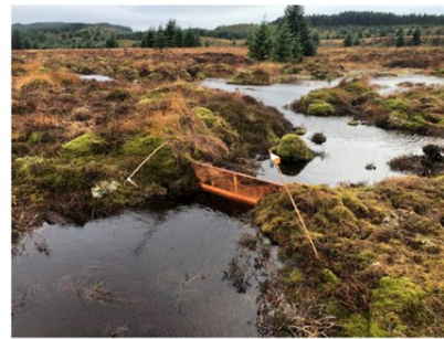
A timber dam used to block a former forestry drain in the vicinity of the Nant Owinau on a forest to bog restoration site in the Cambrian Mountains, with the intention of raising the water table of the surrounding peat.
