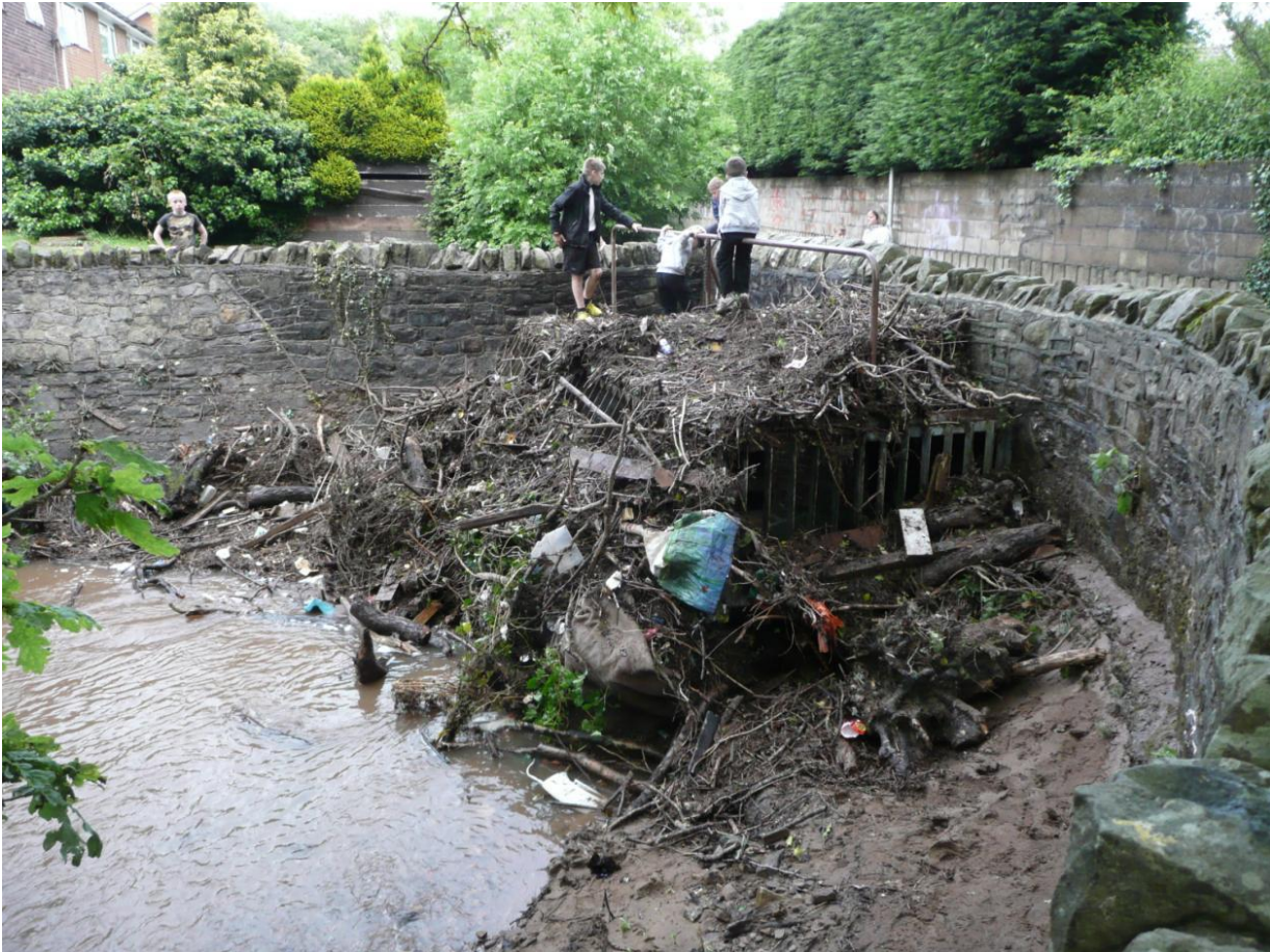
Figure 12. Flooding in Cwmbran in May 2014
