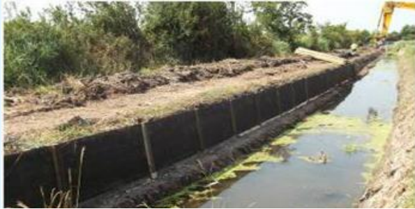
Figure 8 Percoed Reen, Wentlooge Level - Bank Stabilisation works July 2013, photo courtesy of Caldicot and Wentlooge Levels IDB
