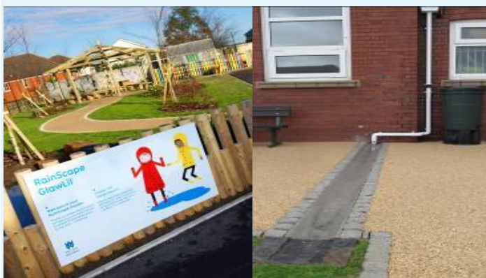
Figure 10 RainScape initiatives at Stebonheath School, photos courtesy of Dŵr Cymru Welsh Water
